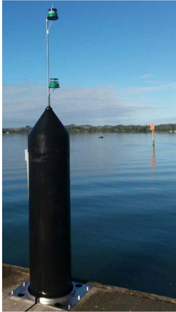
Marina Approach Navigation Lights
